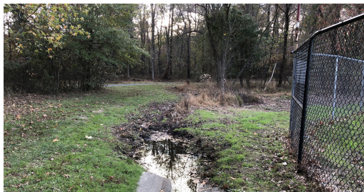
Drainage issues on site
